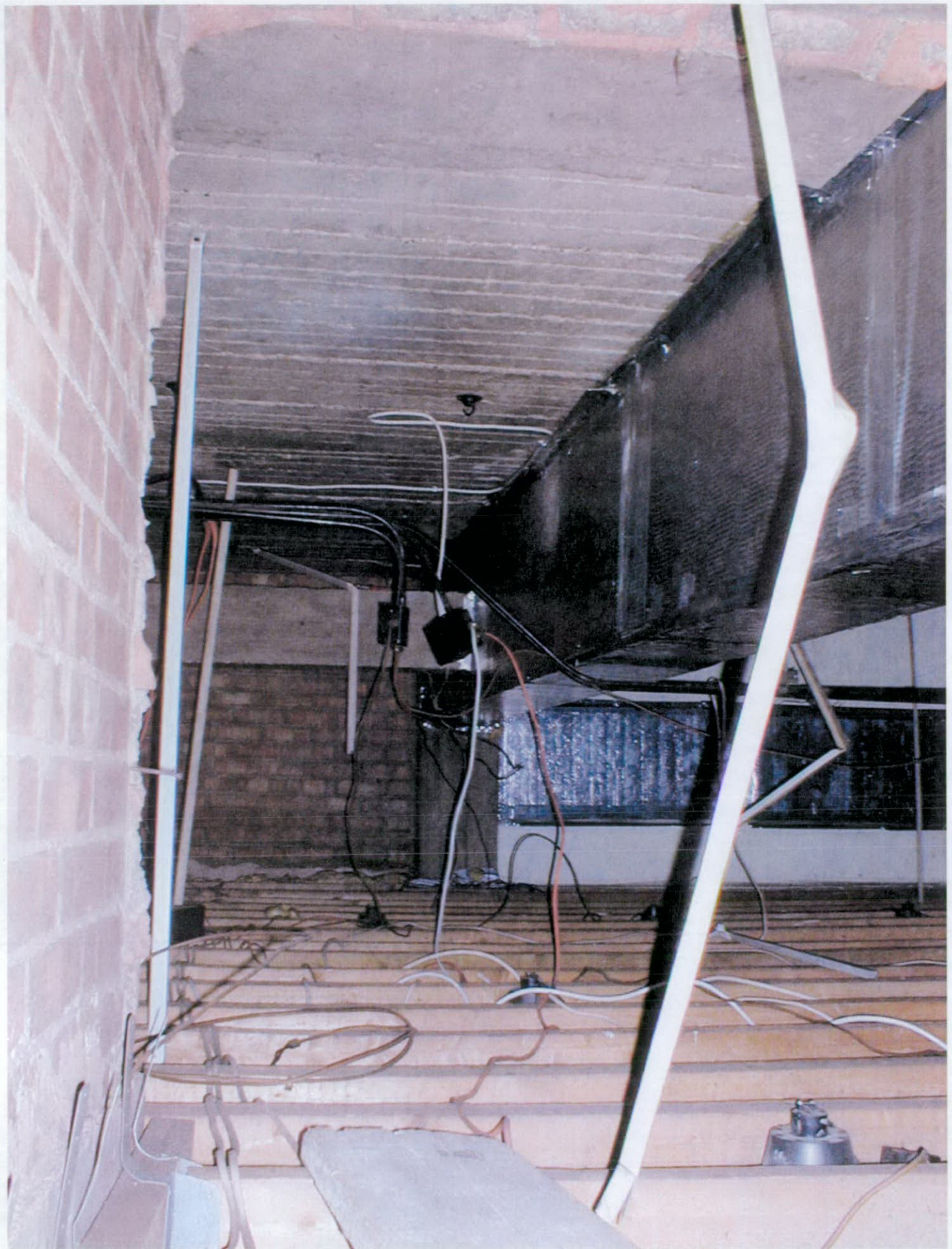
PHOTOGRAPH ABOVE FOYER CEILING SHOWING BRICK PIER ON LEFT (COMMON BRICK), CONCRETE SOFFIT AND BEAM. GATE CINEMA NOTTING HILL PAVLER HUDSPITH
