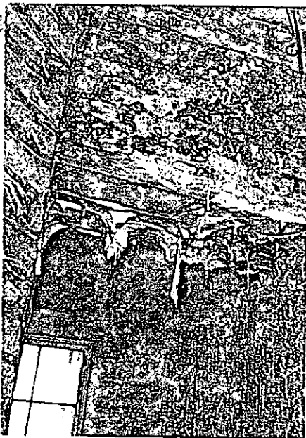
Non-destructive techniques should be used to eradicate dry rot. Adequate ventilation is essential
