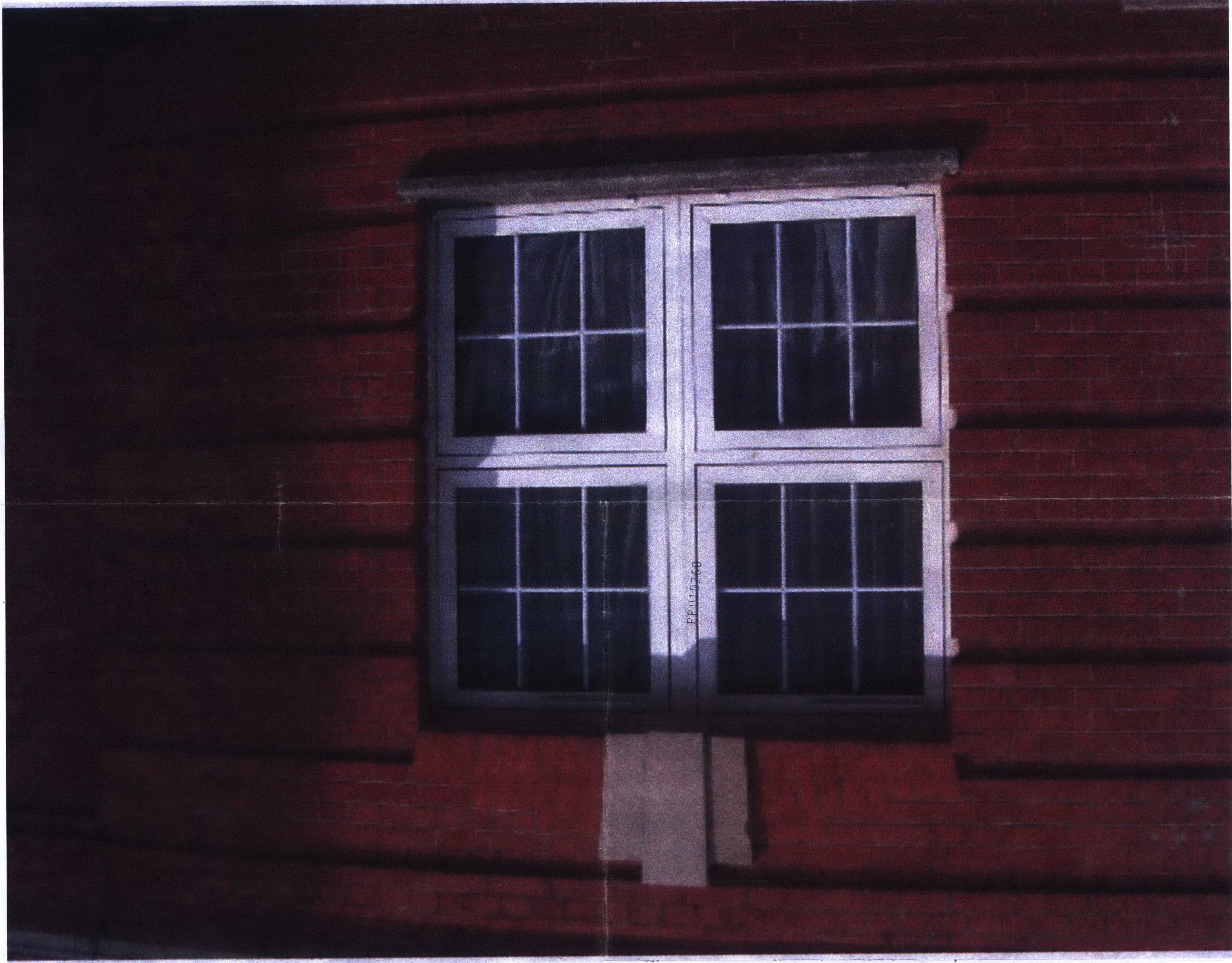
Replacement windows as installed in 1998 to Catwell House, adjacent to Jenningsbury and Kingsmill House.
