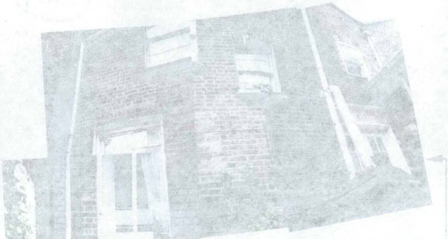
French door of adjacent property onto terrace which extends into party wall, and visible level post of timber staircase which runs from the terrace to the patio and against the party wall.
