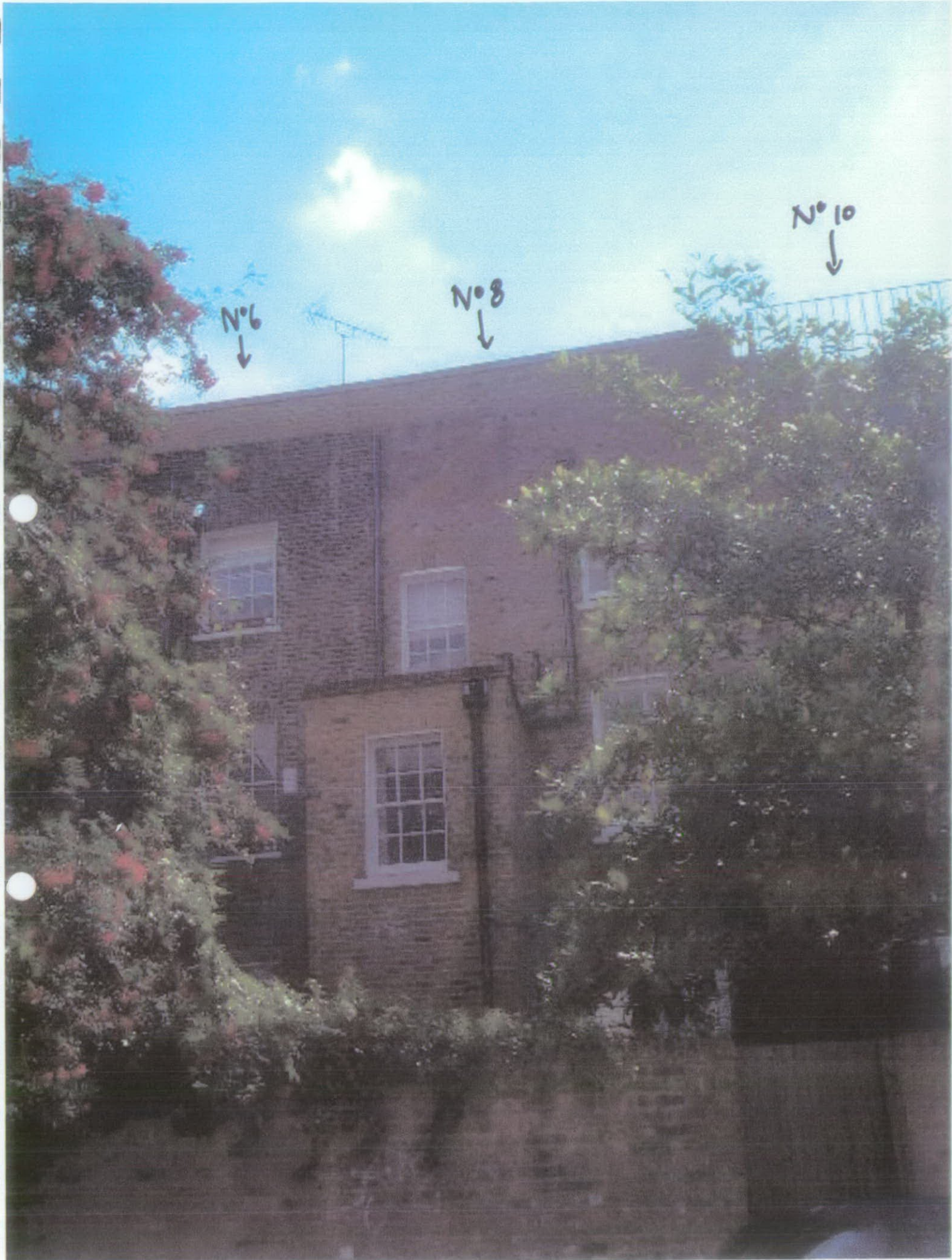
Rear elevation of Nos 6, 8, 10 Penzance Place. Existing structure not visible from road after addition of 525mm to height of rear wall.
