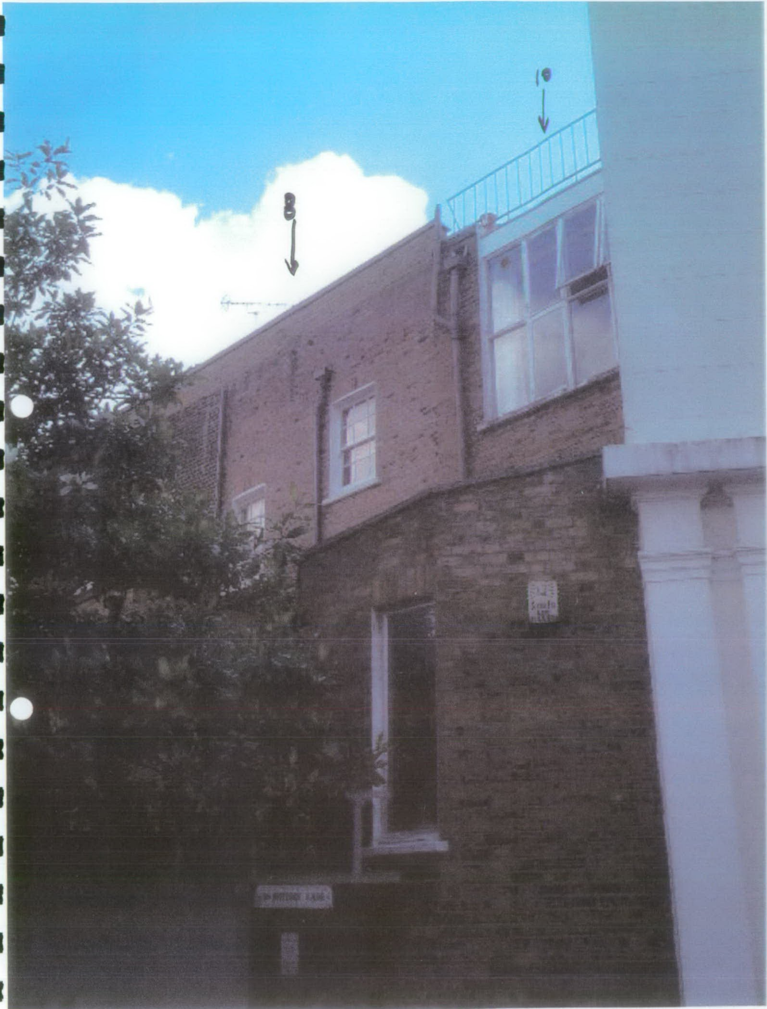
Rear elevations of No's 8 & 10 Penzance Place. Neither are original. Note existing roof structure not visible after additional 525mm added to height. Also inappropriate rear fenestration next door.
