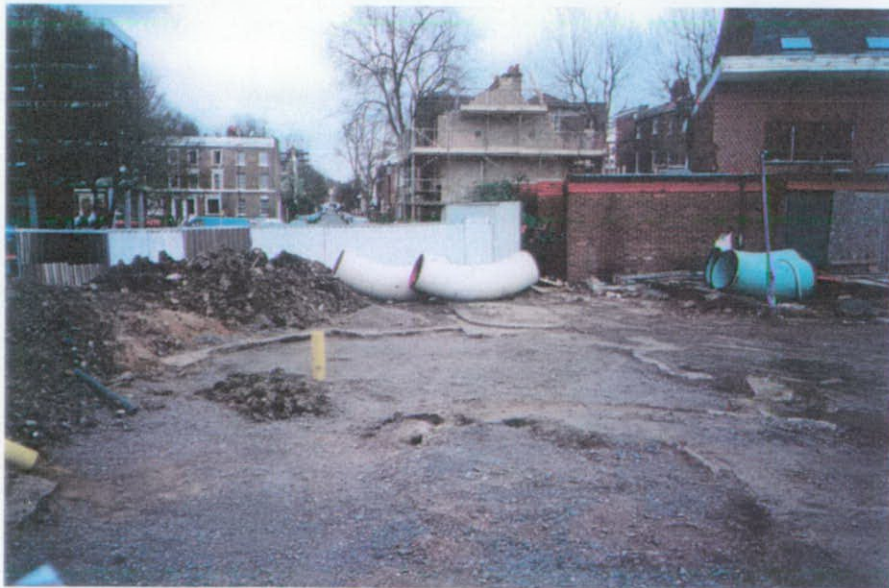
View eastwards across the Appeal Site with the now demolished Sheepshank Public House in the foreground and to the right of the picture
