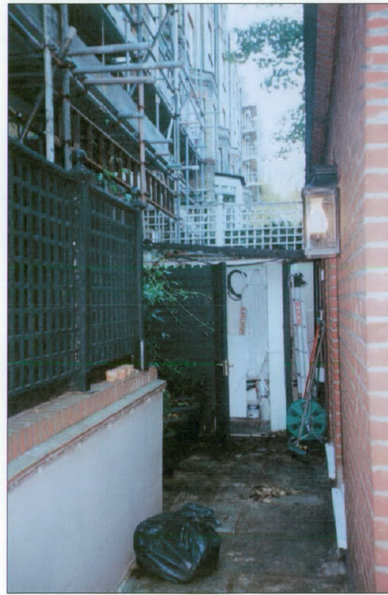
Existing Party Wall Condition - Cranley Gardens
