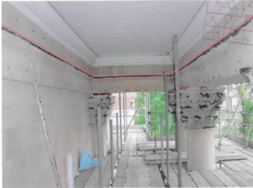
VIEW OF UNDERSIDE OF PORTICO FROM NORTH extent of proposed anti pigeon spikes indicated by red line
