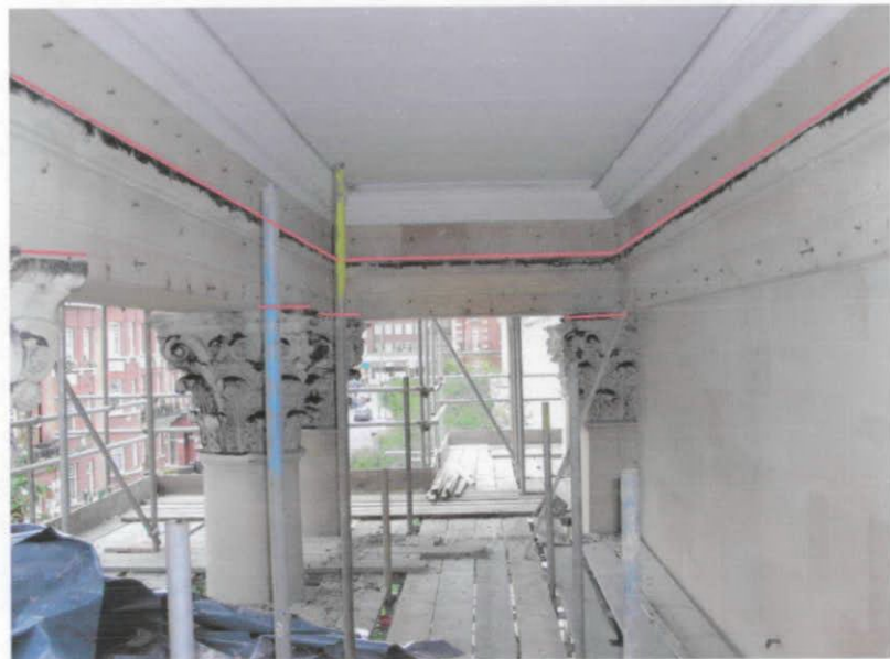
VIEW OF UNDERSIDE OF PORTICO FROM SOUTH extent of proposed anti pigeon spikes indicated by red line
