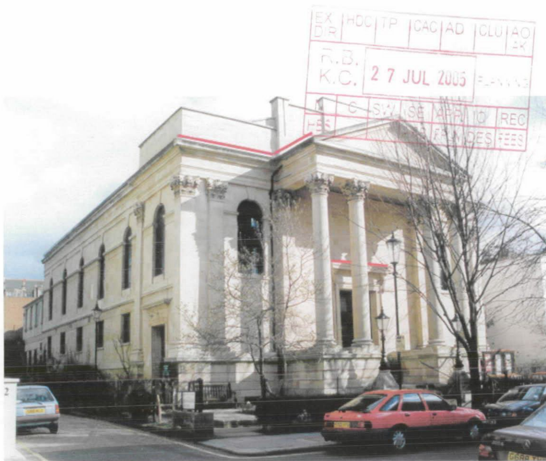
VIEW OF CHURCH FRONT ELEVATION FROM ALLEN STREET & SIDE ELEVATION ALONG ADAM AND EVE MEWS extent of proposed anti pigeon spikes indicated by red line
