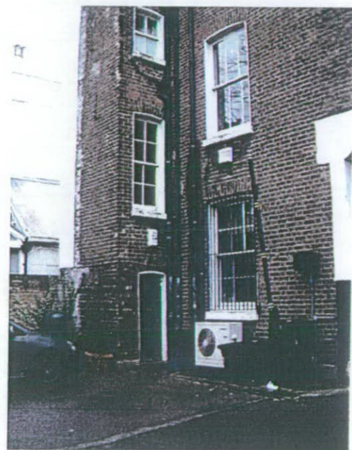
No. 48 Fulham Road - rear access to be relocated from the side to the rear facade
