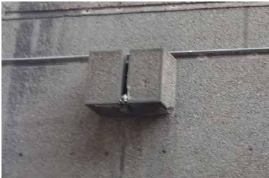
7. Drainage overflow - HTL 2015
