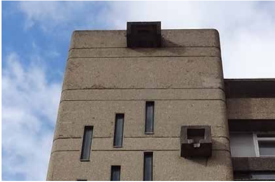
5. Floodlight and extract grille hoods - HTL 2015
