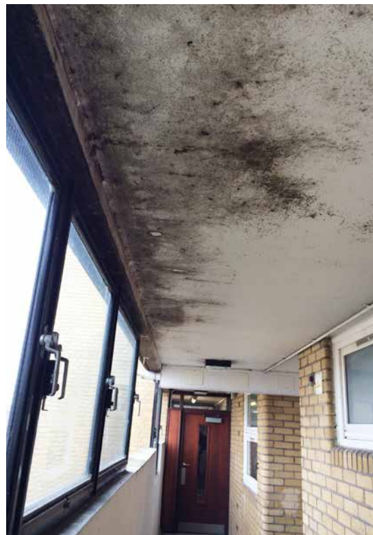
9. Damp to access galleries - HTL 2015
