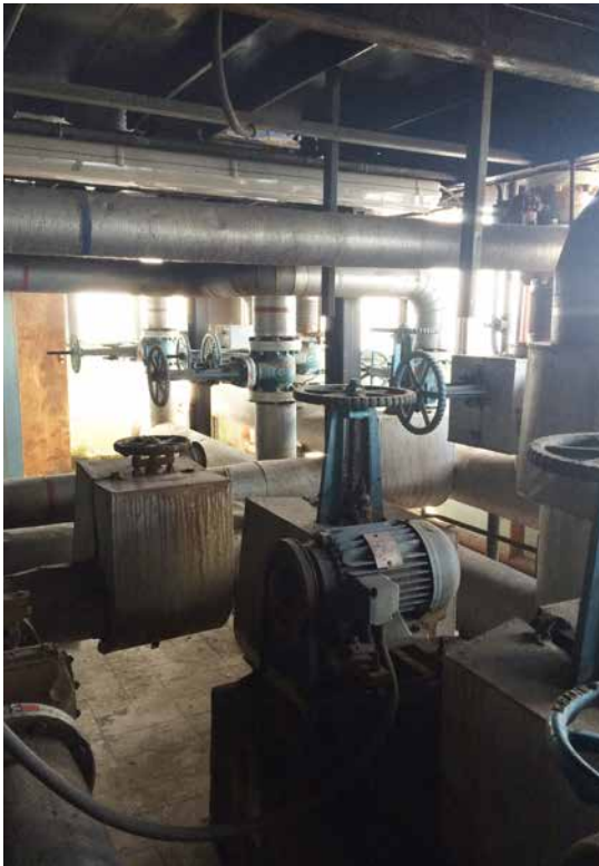
1. Boiler room interior - HTL 2015
