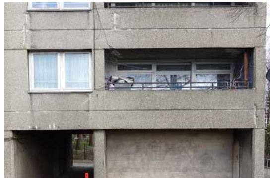
10. Example of localised damage + repairs - HTL 2015
