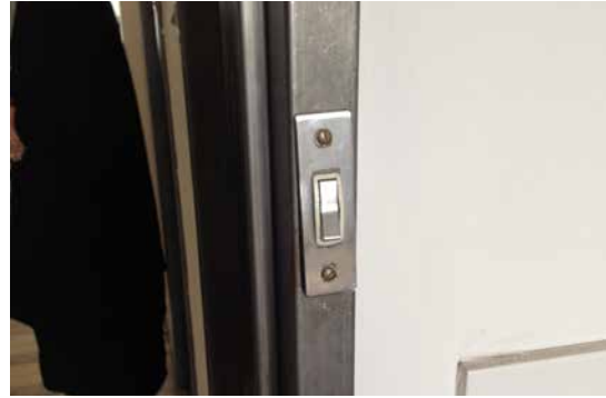
12. Switch integrated into door frame - HTL 2015
