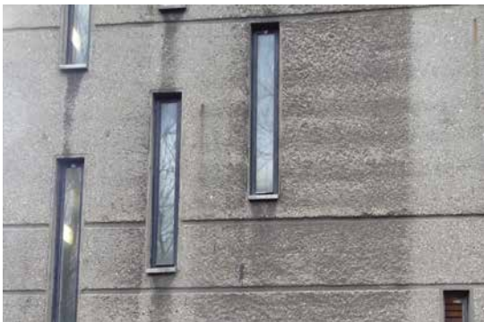
9. Typical staining - HTL 2015
