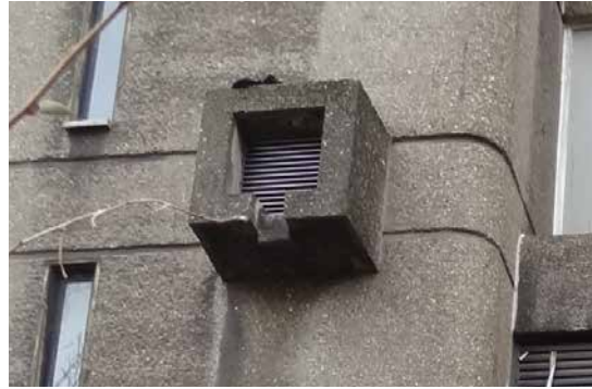
6. Detail of extract grille and hood - HTL 2015
