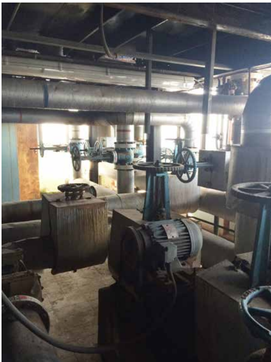
2. Boiler room - HTL 2015
