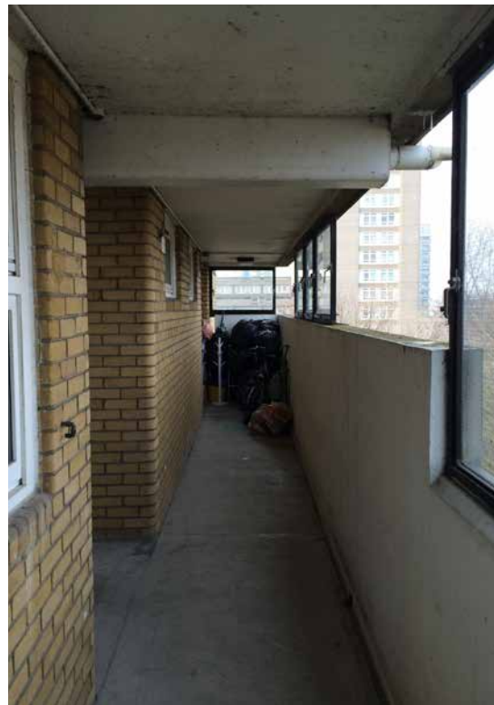
3. Boiler flues to external walkways on block E - HTL 2015
