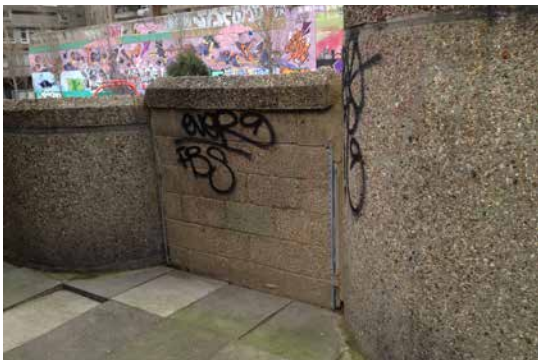
5. Blocked off entrance to ball court stair - HTL 2015
