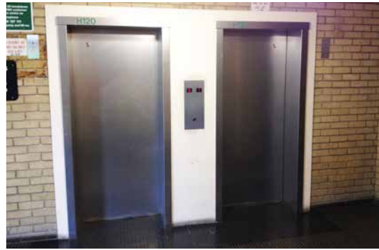
2. Lifts at ground floor - HTL 2015
