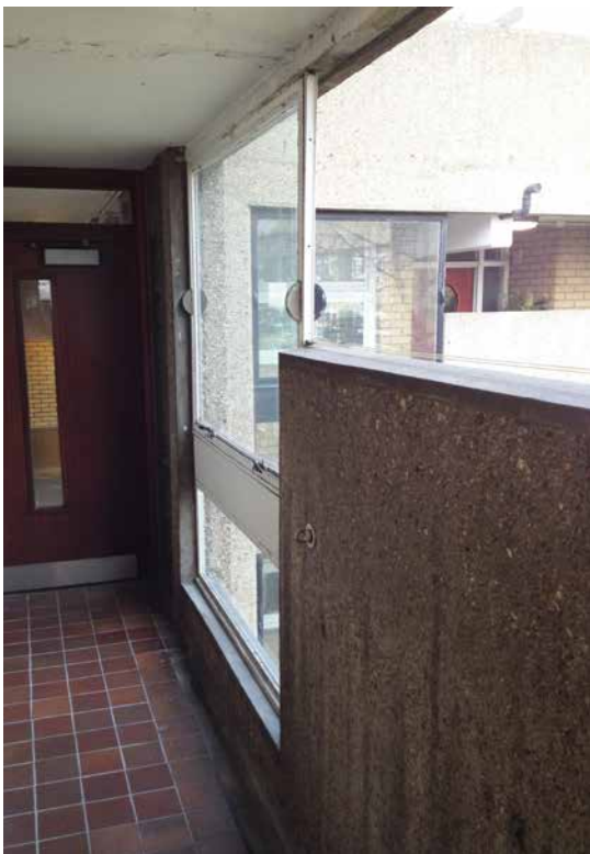
9. Damp visible to access gallery soffit - HTL 2015
