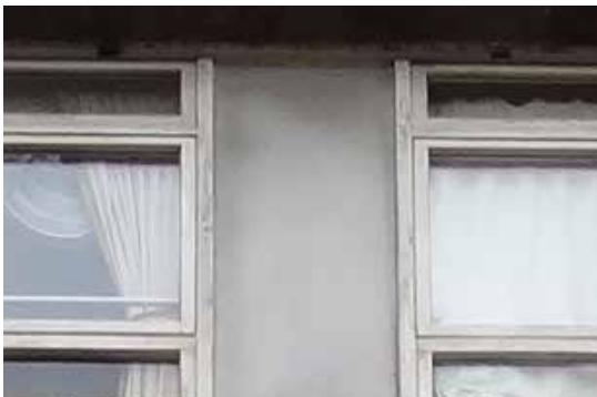
11. Staining to metal faced spandrel panels - HTL 2015
