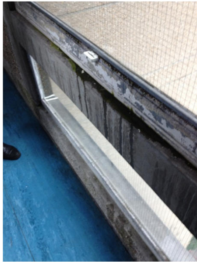
Photo 29 – Evidence of water ingress to communal window
