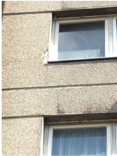
Photo 25 – Concrete disrepair example
