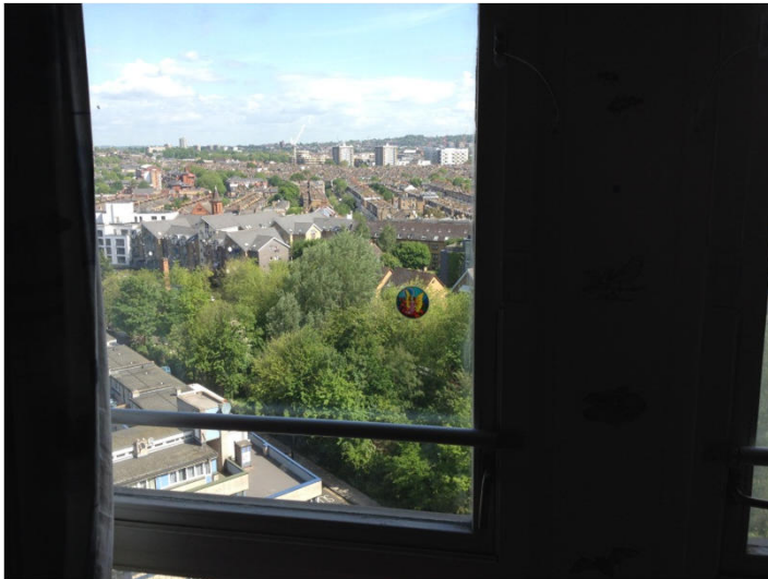
Photo 9 – Bar restrictor to north elevation window
