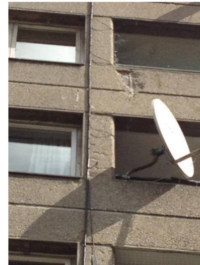
Photo 24 – Concrete disrepair example
