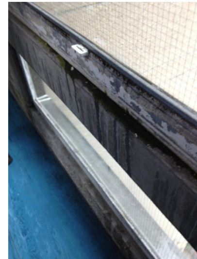
Photo 28 – Evidence of water ingress to communal area link bridge window
