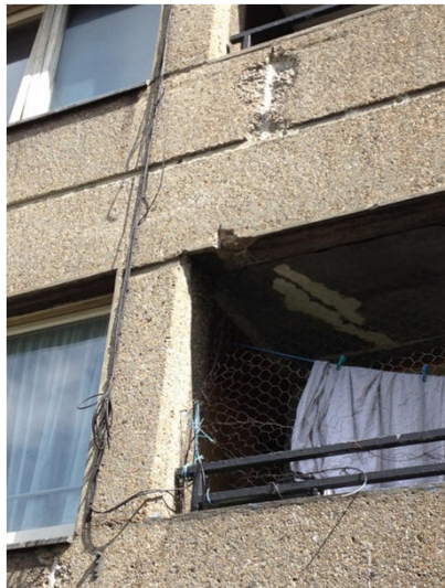
Photo 23 – Concrete disrepair example
