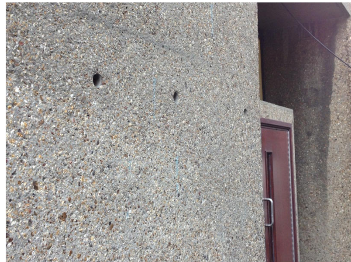
Photo 20 – Blown concrete to reinforcement
