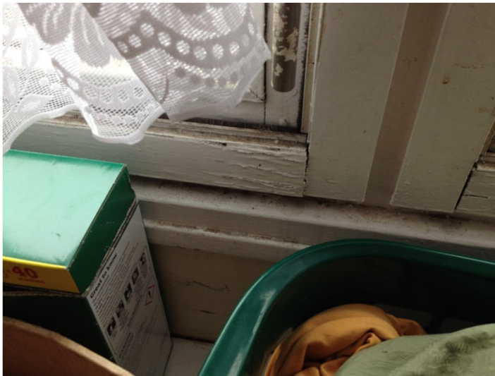
Photo 27 – Timber decay to kitchen window
