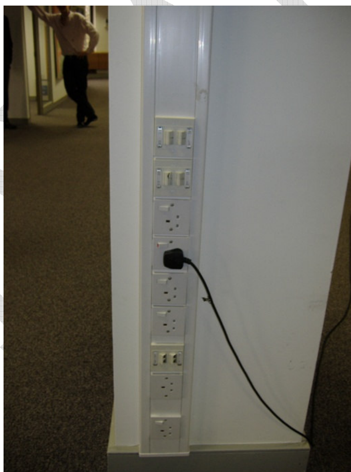
View of Tenants Improvised Power Trunking (building has no raised floor)
