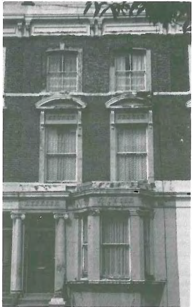
Decaying stucco, broken mouldings, painted brick and trailing wires: Chesterton Road
